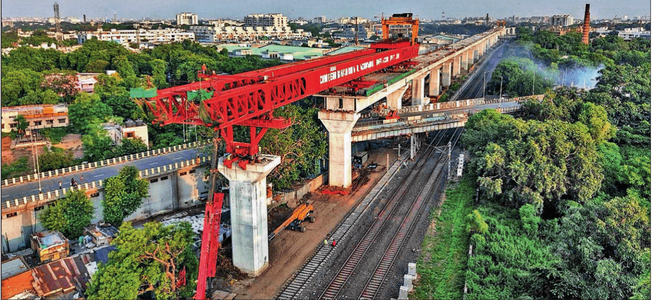
The Girdharnagar bridge, a component of the Mumbai-Ahmedabad bullet train project, was completed in just 12 days by the National High-Speed Rail Corporation Limited. The bridge, a 45m-long viaduct, was launched over the railway flyover on the Delhi-Ahmedabad main line
