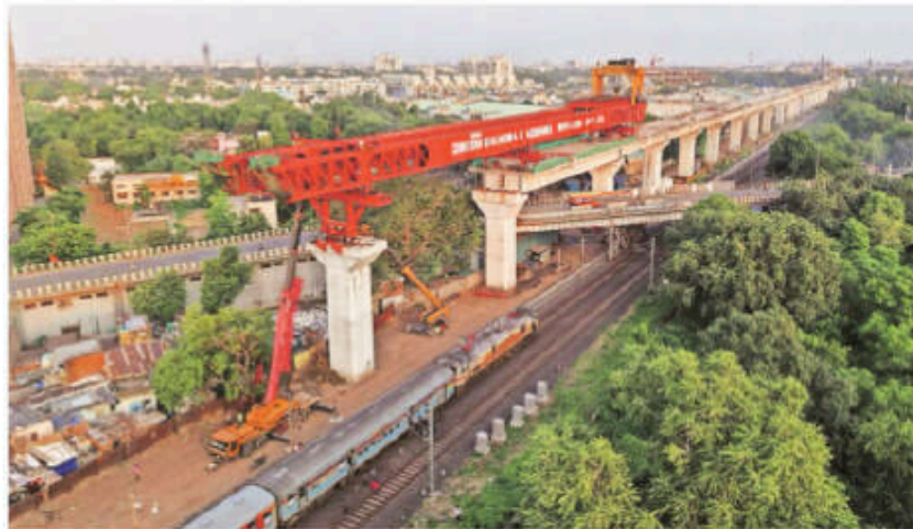
19 segments launched to complete the 45-metre span of the viaduct that runs parallel to the existing railway line in Ahmedabad. Pic courtesy: NHSRCL
